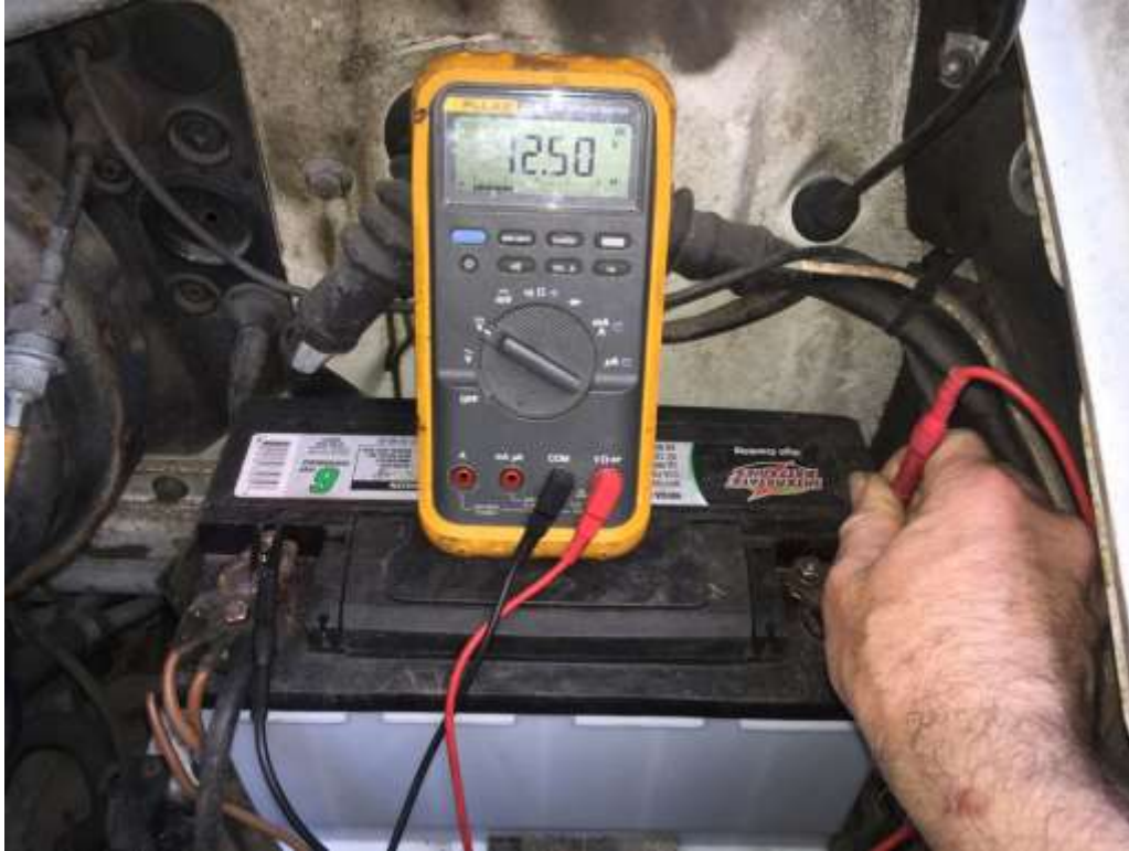
Using a multimeter to measure battery voltage. This one is a tad low.
