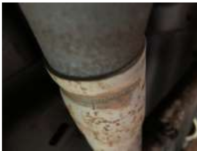
Picture 3. Result of an over-tightened clamp.
